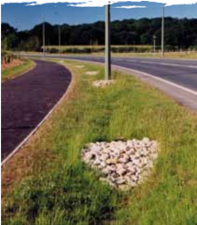
Witney, Oxfordshire – a stone check-dam in a roadside swale to slow flows and prevent erosion. Stones that become hidden in grass may pose management risks. Photo: Bob Bray
